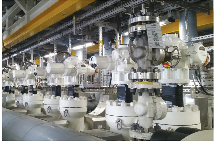
Rotork intelligent actuators have been installed on the all-electric Johan Sverdrup platform
