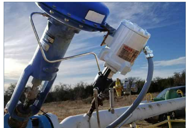
PAX 1 installed as a pilot on a natural gas Control Valve
