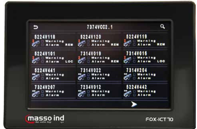
2. VALVE LIST with Feedback and Warnings/Alarms status
