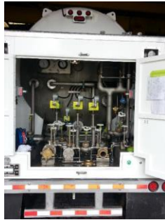
Schischeck ExMax on an LNG transportation tanker
