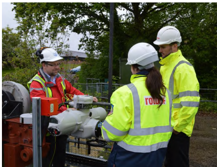
IQ3 actuators at a water treatment plant in the UK
