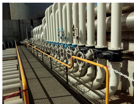
IQ3 actuators at a tank farm in Spain
