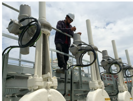
An engineer checking the commissioning settings on an IQ3 at a storage tank facility in Malaysia
