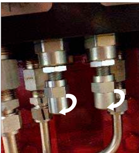
Fig 12.6 Flow regulator cap removal
