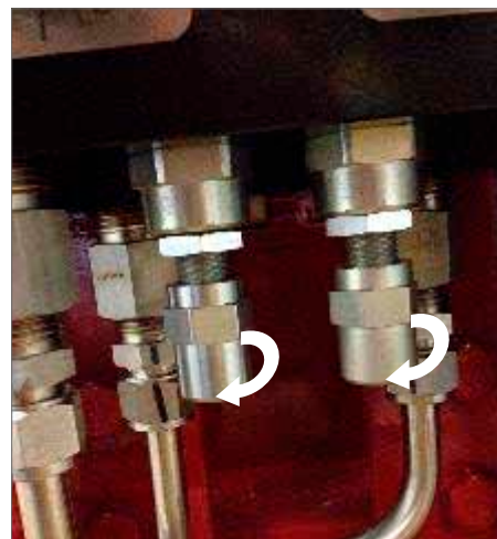
Fig 11.4 Flow regulator cap removal
