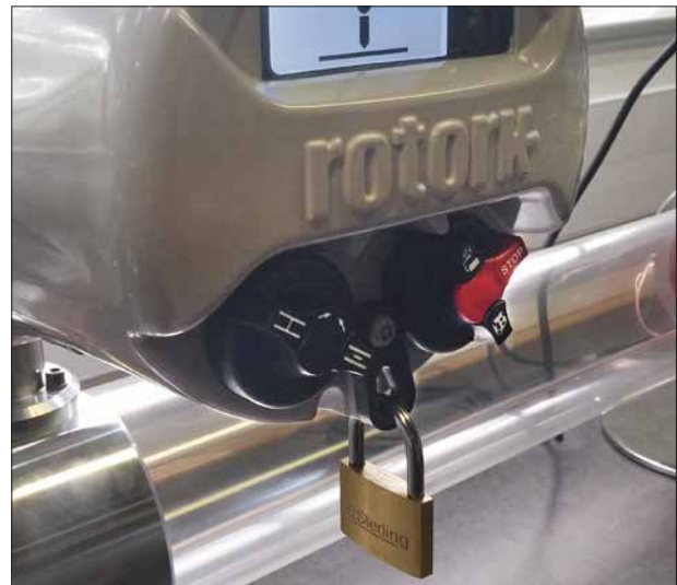
Fig 7.2. IQ3 control selector padlocked in "Remote"
