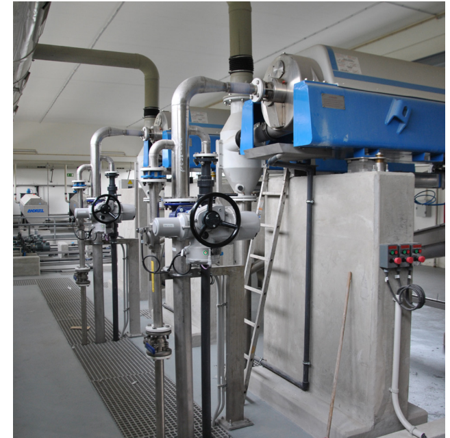
Above: Profibus DP enabled Rotork non-intrusive IQ intelligent valve actuators installed at the Viseu Sul WWTP in Portugal, described as a national environmental benchmark for future developments.
