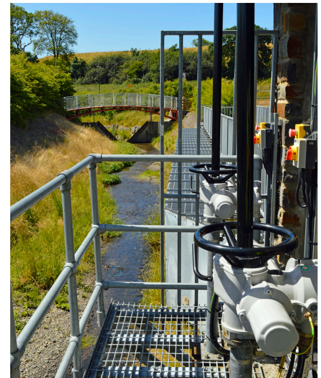
Above: The River Mwidan flood alleviation scheme, showing two of the new Rotork actuators in the foreground and the V notch weir in the background. The over-spill grid is in between.
