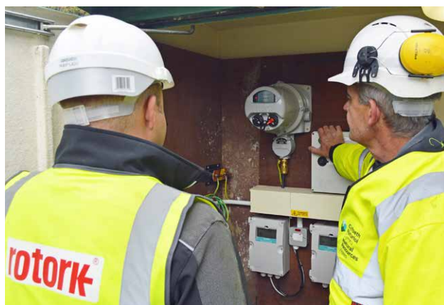
RHS operating SI range actuators in inaccessible locations
