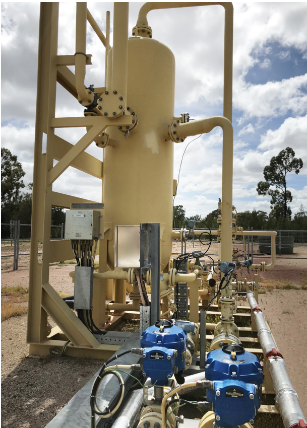
Figure 1. Rotork CVQ electric actuators operate valves on separator skids at an Australian onshore natural gas site.
